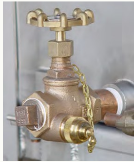
Drain Valve with Sampler
