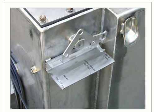
External Ground & Relay Cut Out Switch
