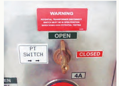
Internal Potential Transformers for Power Calculations and Control Power
