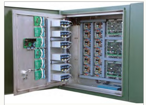
Custom Automation and Relaying Controls for Smart Grid Applications
