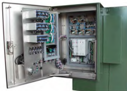
Customer Specified RTUs Combined with SEL Over Current Control
